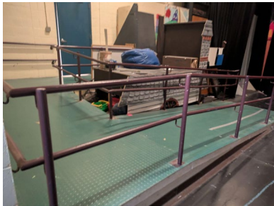
Cumbersome and difficult-to-find ramp to Wood Gym does not include lighting at the top of the ramp.
